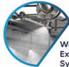
FM200 Fire Extinguishing System
